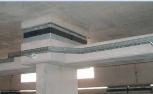
Spring support in underground car park
